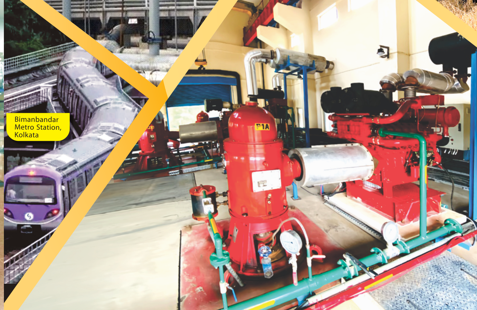
Storm Water Pump House - OWSSB, Orissa
