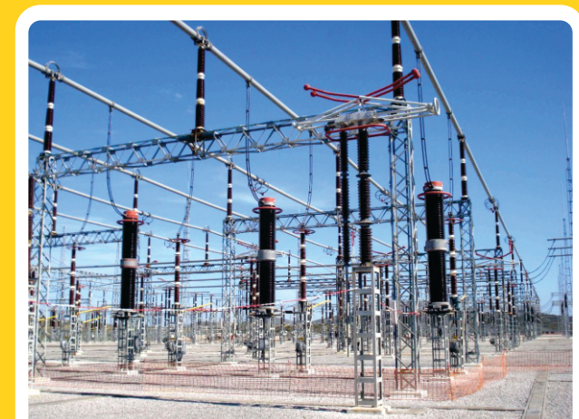
Sub Station at Serum Institute of India Ltd, Pune
