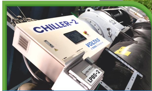
23000 TR Chillers in Tata Solar Module Mfg. Unit
